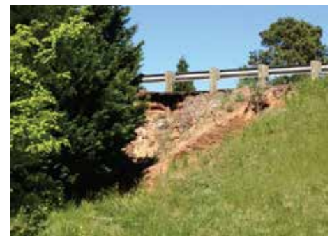
Severe slope erosion
