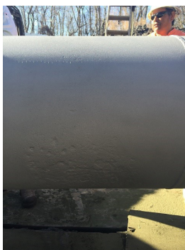
View of corrosion
